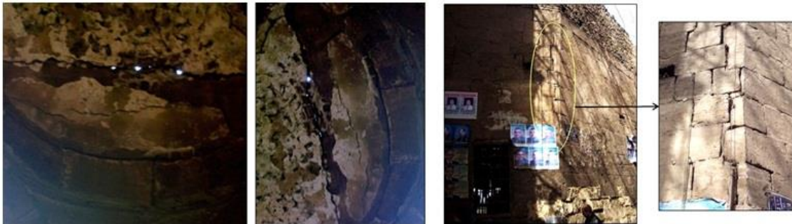
Figure 13: Active vertical cracking in dooms and perpendicular walls connection region
