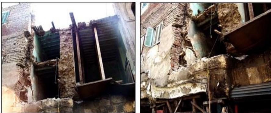
Figure 7: first floor in destroyed current situation.
