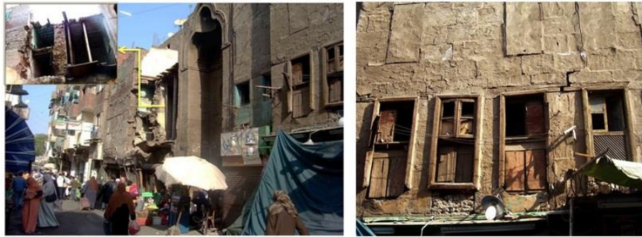
Figure 10: Out-of-plan-failure and cracking in wall 1
